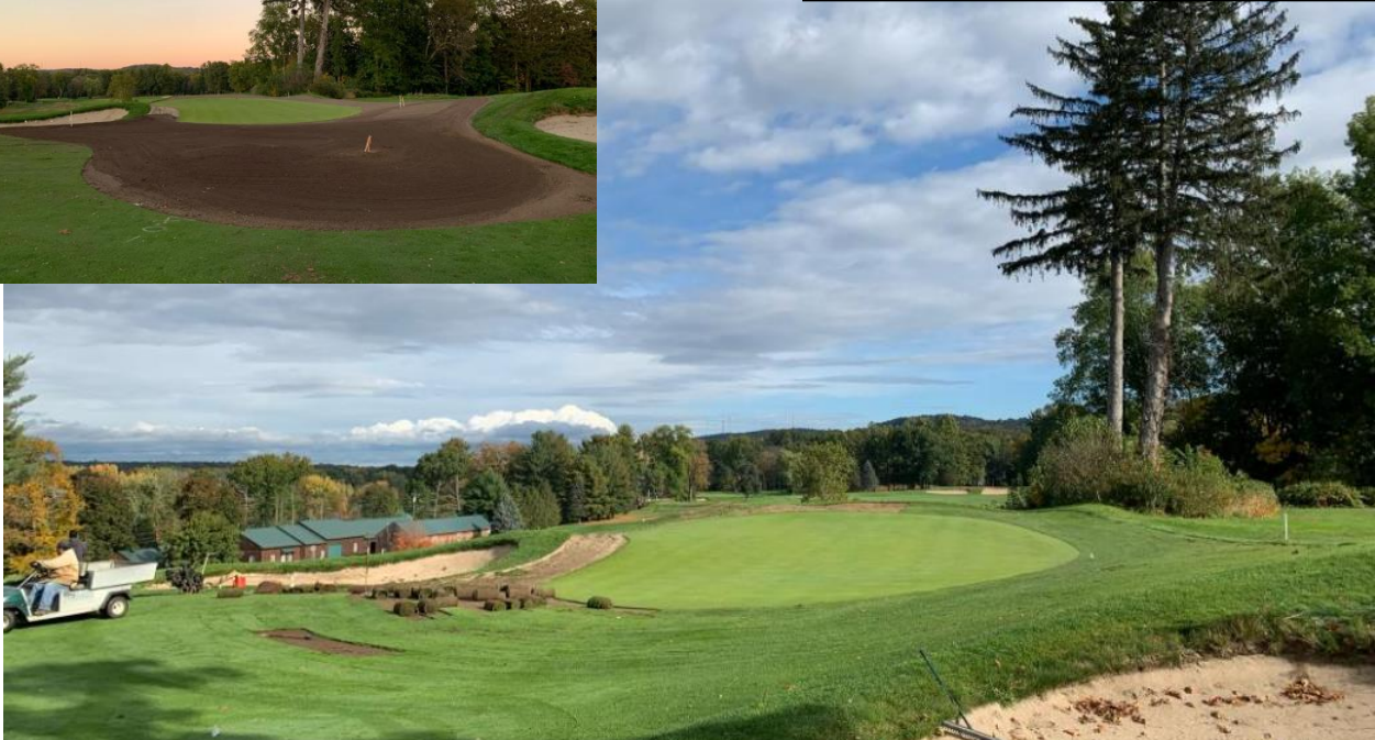
View of CCF's first green as the expansion process was beginning. Inset photo shows the regraded approach which resolved a perennial drainage issue and created a distinct ground contour to add variety. Photos: Matt Dusenberry
